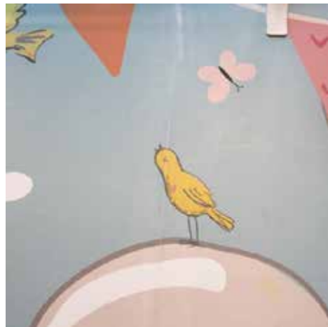
Wallpaper already scuffed during installation
